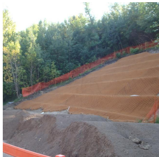
Tough Cell® installed
