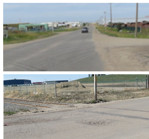
Top: Completed road after 1 year of operation Bottom: CTB section left of crossing shows cracking
