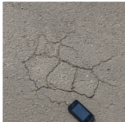
Fatigue cracking in road surface before construction
