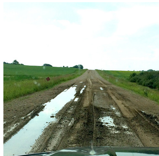
Roadway conditions after heavy rain
