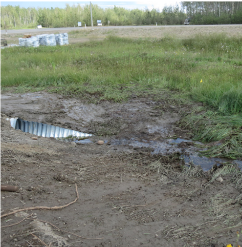
Mud and drainage issues before construction
