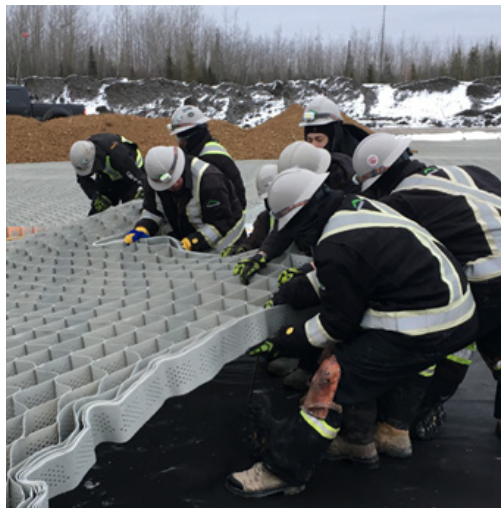
Tough Cell® installed
